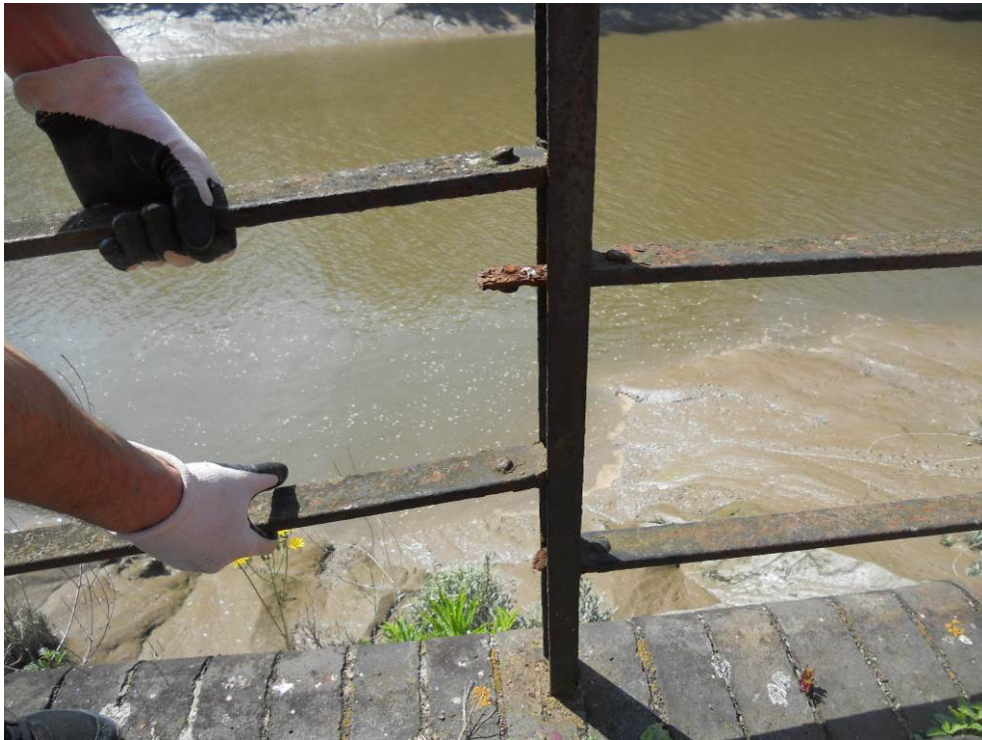
Photo 13 – Corroded Fixings to Intermediate Rails (Ch210m)
