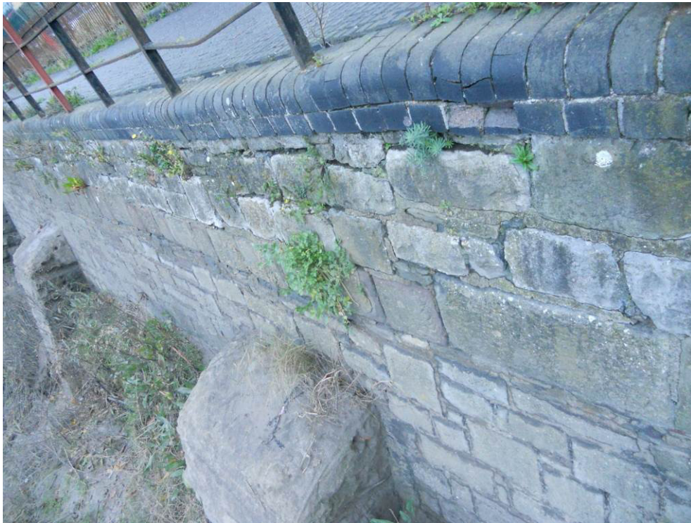
Photo 09 – Mortar Deterioration above Buttress B17 (Ch180m)
