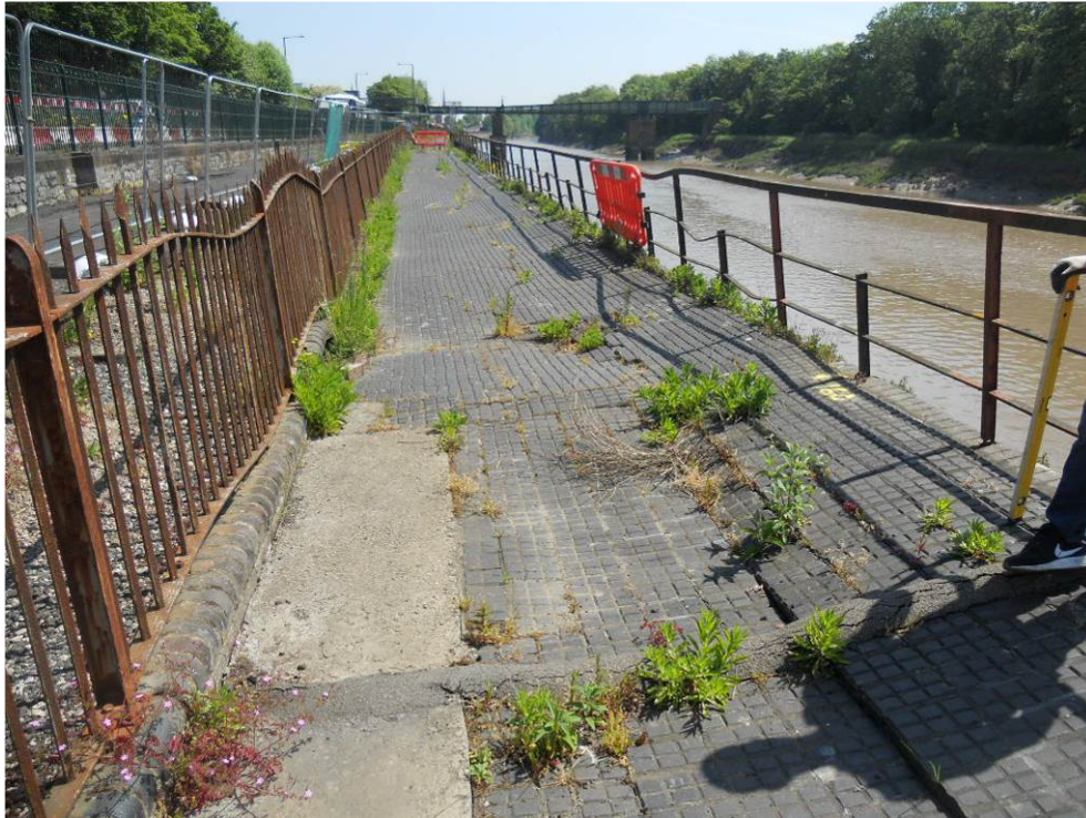
Photo 17 – Major Deformation of Chocolate Path (Ch160m)
