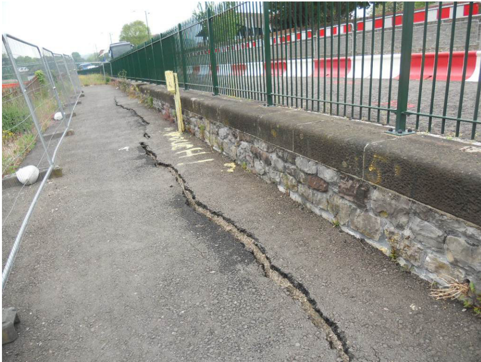
Photo 21 – Tension Crack in Tarmac over Railway (Ch147m – 195m)
