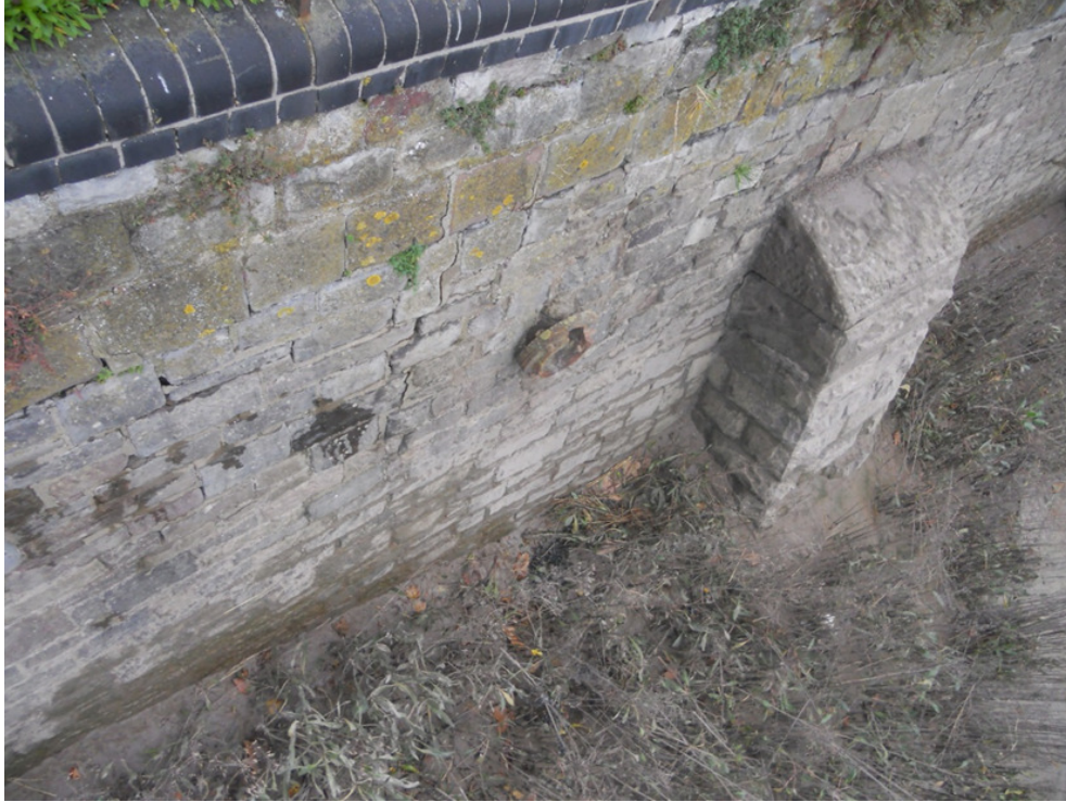
Photo 05 - Cracks in Wall Near to Buttress B11 (Ch144m)
