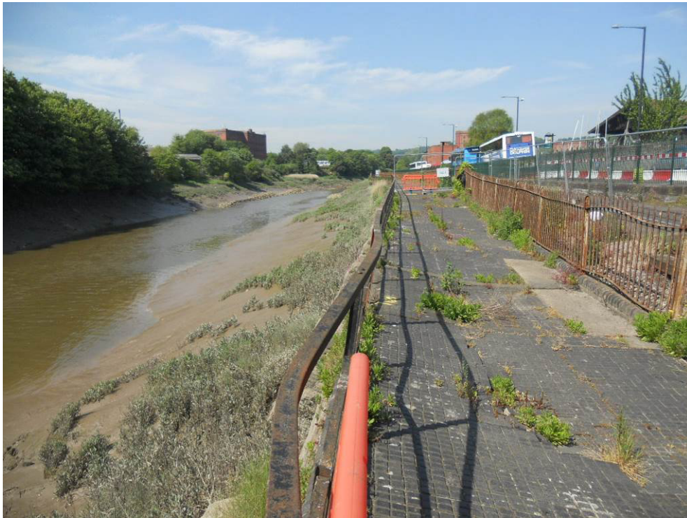
Photo 11 – Major Distortion of Railings at Centre of Slip (Ch170m)
