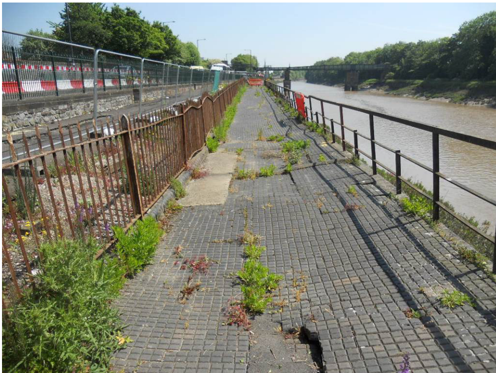
Photo 18 – Major Deformation of Chocolate Path (Ch150 - 160m)
