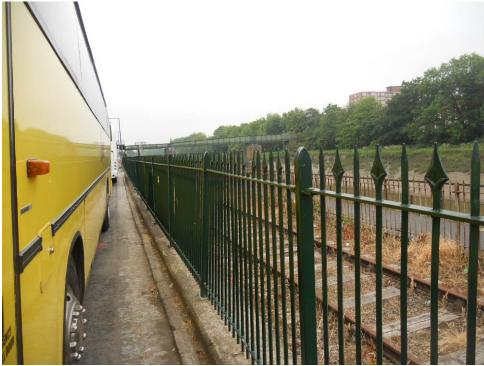
Photo 25 - Cumberland Road Railings – Minor RTA Damage to 3 Panels (Ch220m)
