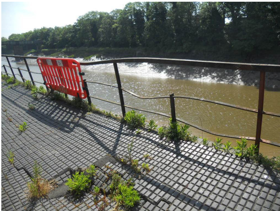
Photo 10 – Major Distortion of Railings at Centre of Slip (Ch170m)
