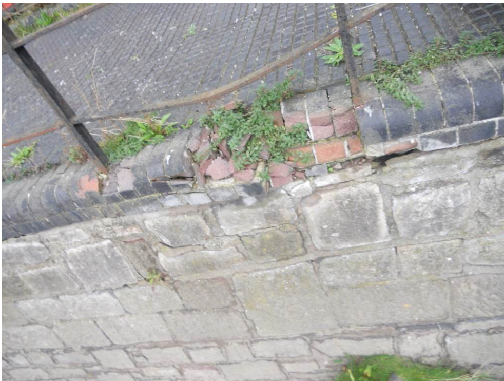
Photo 08 – Displaced Brickwork Above Buttress B15 (Ch168m)
