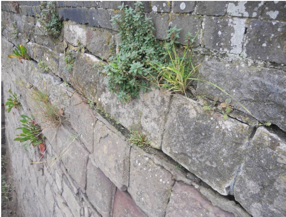
Photo 07 – Displaced Stonework Between Buttress B13 and B14 (Ch157m – 160m)
