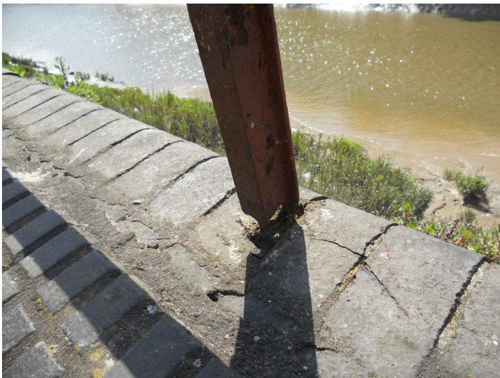
Photo 12 – Localised Severe Corrosion to Base of Parapet Post (Ch140m)
